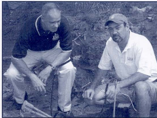
Dale Kuhn (JULIE, Inc.) and Art Kraus (Kraus Cable TV) inspect a damaged communications line that was not reported.
